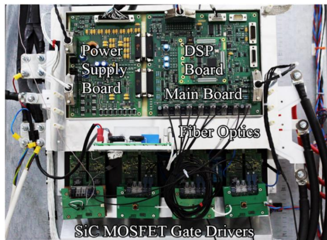
Figure 3.28. Final assembly of the power electronic block
