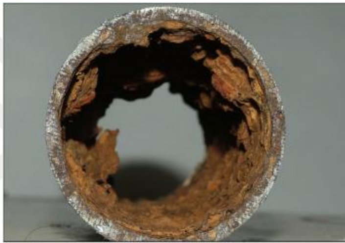
Figure 1.7 Corrosion and scale effect (16).
