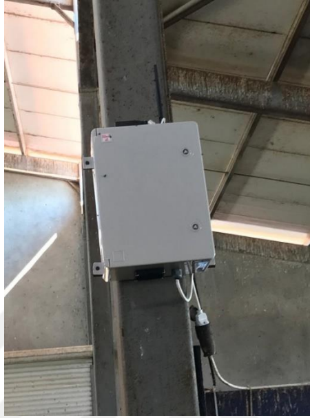
Figure 23: Overview of the air quality monitoring system installed in a dairy barn
