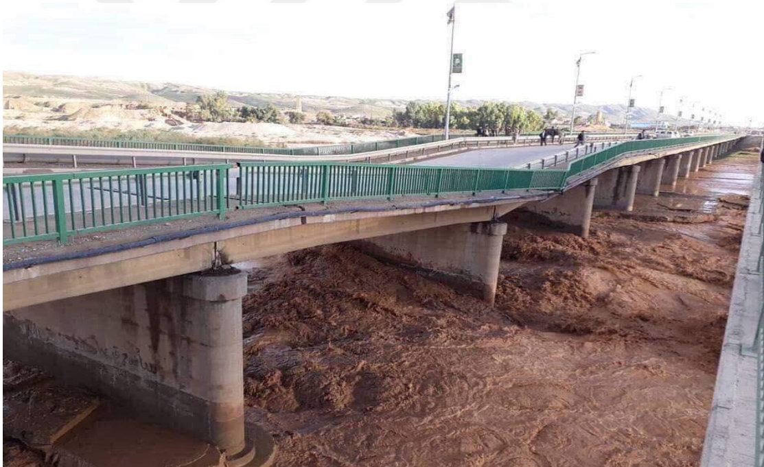
Figure 1.1 Failure of settlement in one of the piers of Tuz bridge in Salahdin.
