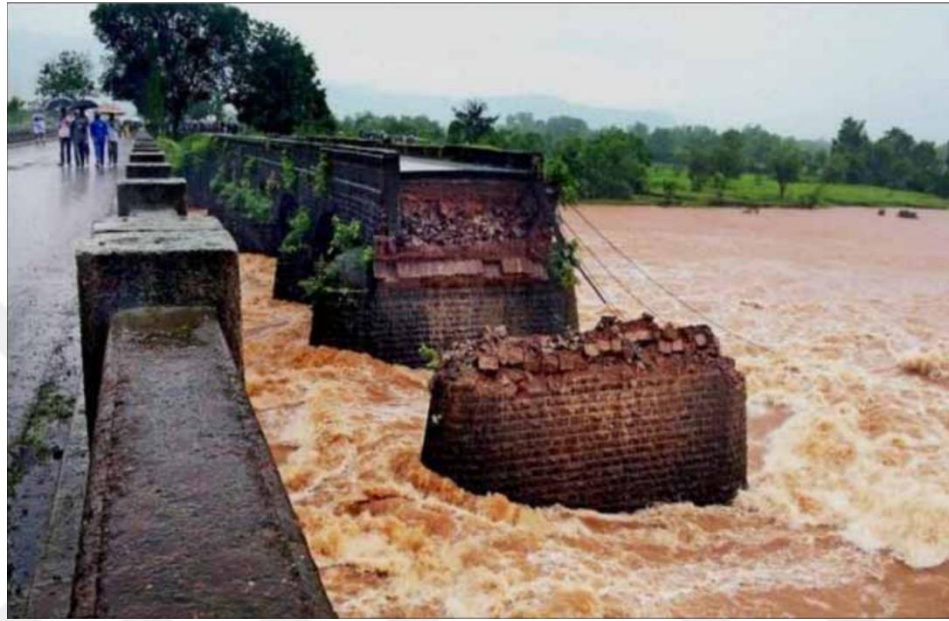
Figure 2.9 Collapsed Bridge, Mahad. Source: Times of India /bridge-collapse-on-goaliveblog.
