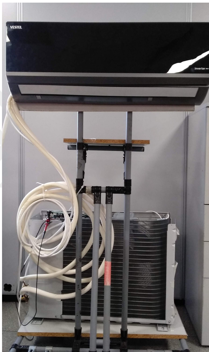
Figure 5.2.2: Air conditioner setup including inverter board with 10uF film capacitor
