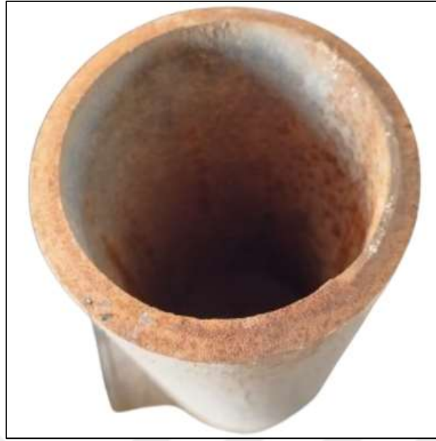
Figure 4.6: Visibly Undetectable Crack in a Pipe Section.
