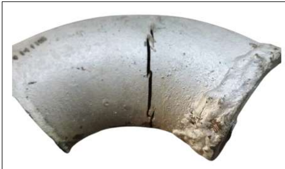
Figure 1.3: Corrosion Crack in a Pipe Section Taken from Beiji Refinery in Salahddin, Iraq.
