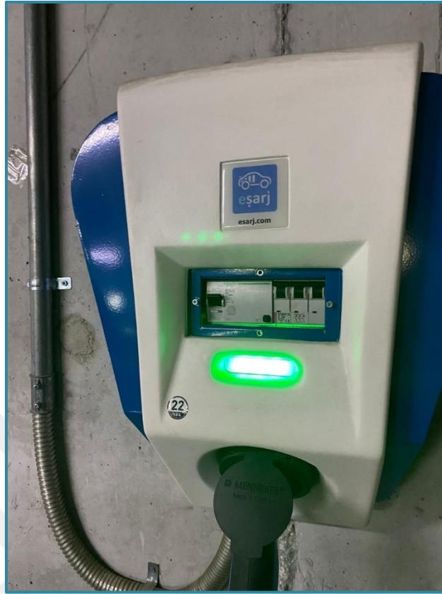
Figure 2.4. Level 2 Charge Station
