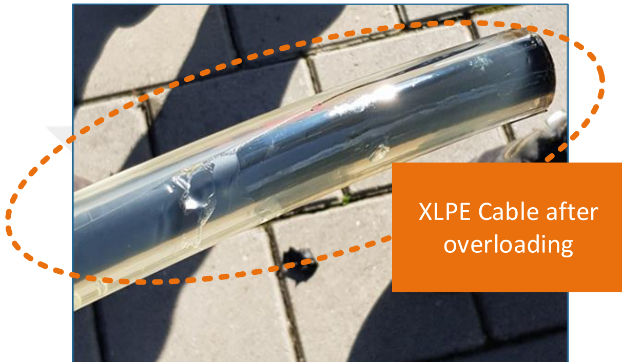
Figure 1.7. XLPE Cable after Overload
