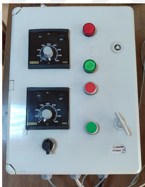
Figure 3.27. Exhaust gas heater control panel
