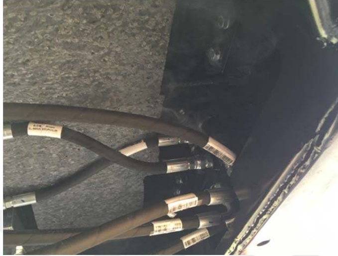
Figure 5.2. Leaking Fog Through Pedal Valve and Operator Foot Restraint Area
