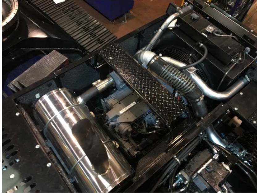
Figure 4.24. The Engine Room Where Polyethylene Sound Absorbers are Installed Visual
