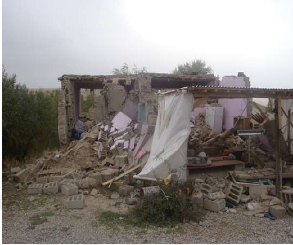
Figure 1.2 Total damage to the masonry house (Taken from the archive of Assoc. Prof. Dr. İdris Bedirhanoğlu, Bedirhanoglu 2011a)
