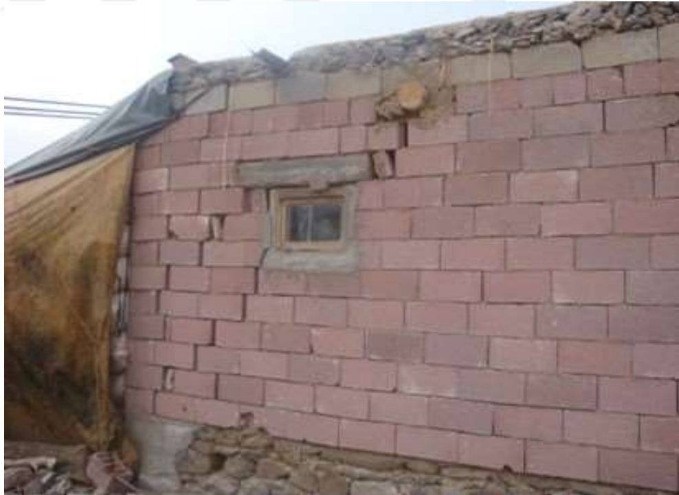
Figure 1.3 Diagonal damage to the masonry house after the Van Earthquake 2011 (Taken from the archive of Assoc. Prof. Dr. İdris Bedirhanoğlu, Bedirhanoglu 2011a)
