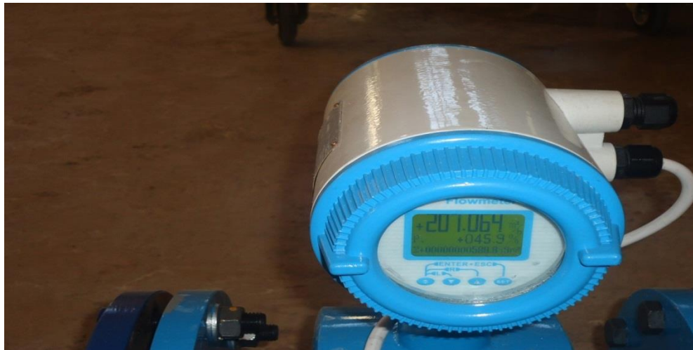
Figure 3.3 Magnetic flow meter installed in the pipe system
