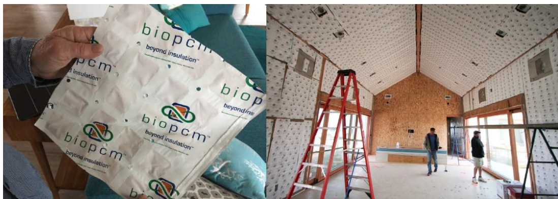
Figure 6.62 Photo of PCM (left image) and its' implementation (right image) [270]
