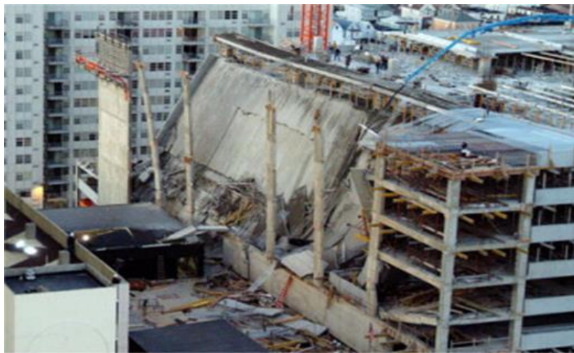
Figure1.1: progressive collapse due to punching of flat slab [3]
