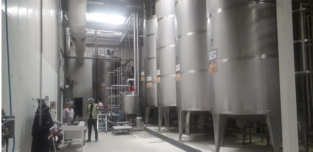
Figure 3.1 Photograph of Syrup Storage Room
