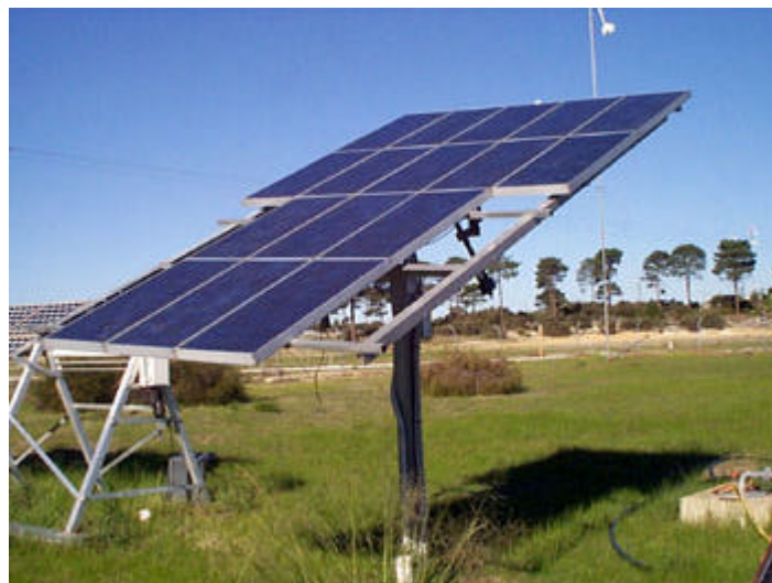
Figure 4.2 Tracked PV Array
