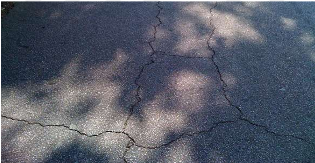
Figure 3.2: Sample of Minor Crack.
