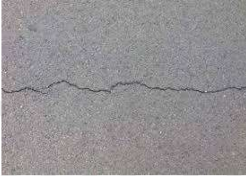
Figure 3.5: Sample of Simple Crack.
