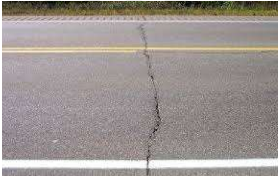
Figure 3.3: Sample of Moderate Crack.
