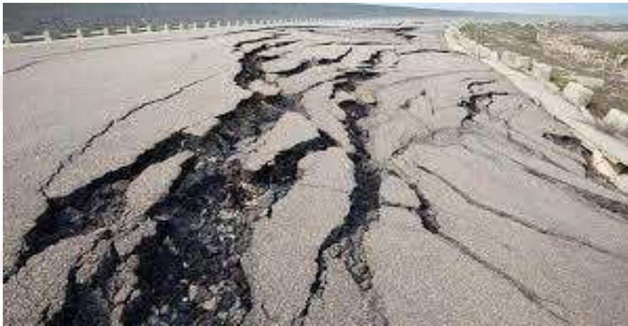
Figure 3.4: Sample of Sever Crack.
