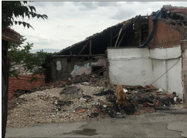
Figure 55: Burned Squatter House in Kale Neighborhood
