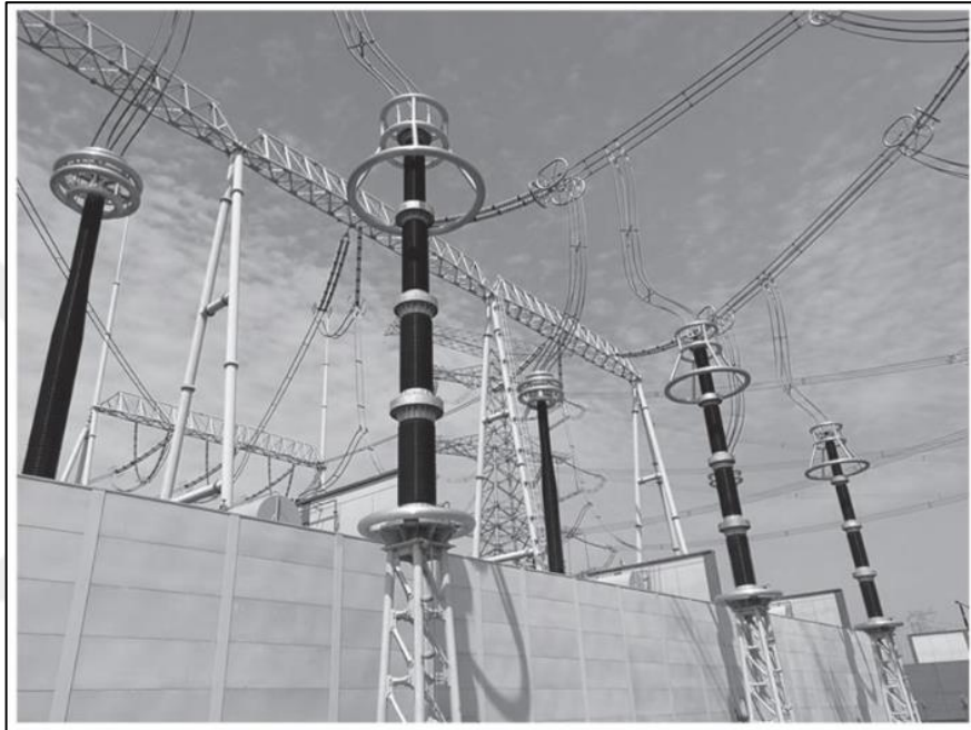
Figure 4.2. 1000 kV ultrahigh voltage AC surge arresters with porcelain houses [95].
