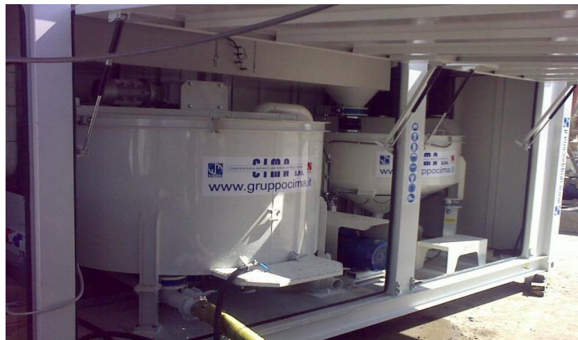
Figure 5.7 Injection preparation unit
