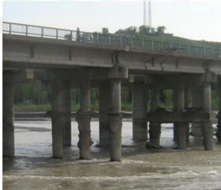
Figure 2.6. The condition of substructure of Filyos Bridge due to scour (Avsar, Atak, & Caner, 2017)
