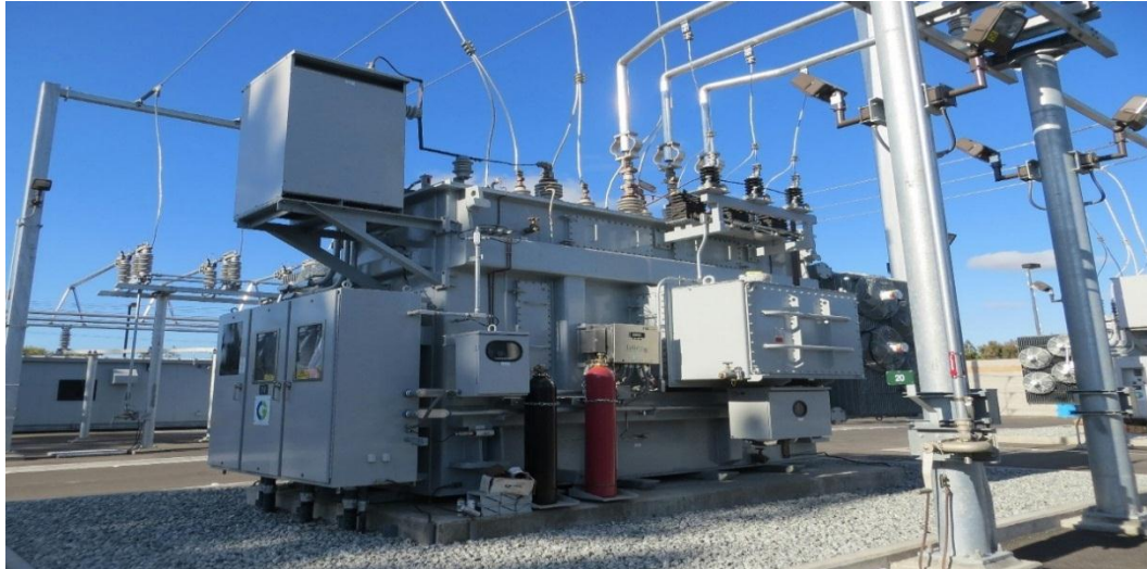
Figure 3.2. Substation 33/11kV for electricity distribution [55].
