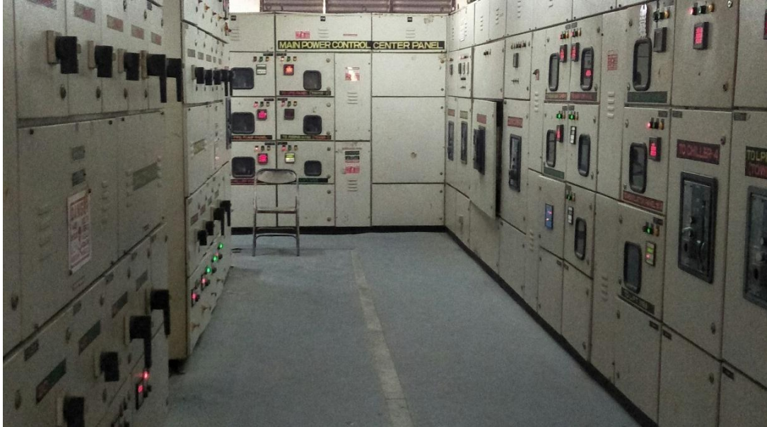
Figure 3.5. 33 kV & 11 kV Circuit breakers [56].
