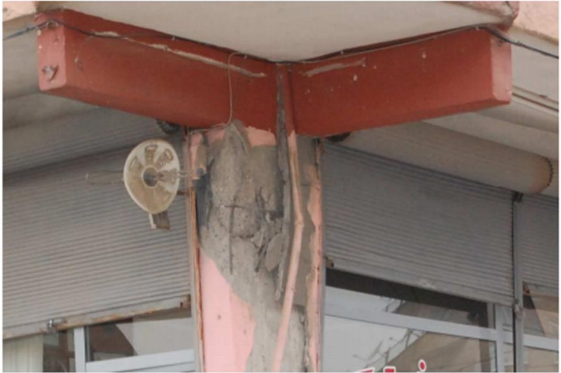
Figure 1.1 Damage to the column under vertical load (Taken from the archive of Assoc. Prof. Dr. İdris Bedirhanoglu, Bedirhanoglu 2011a)
