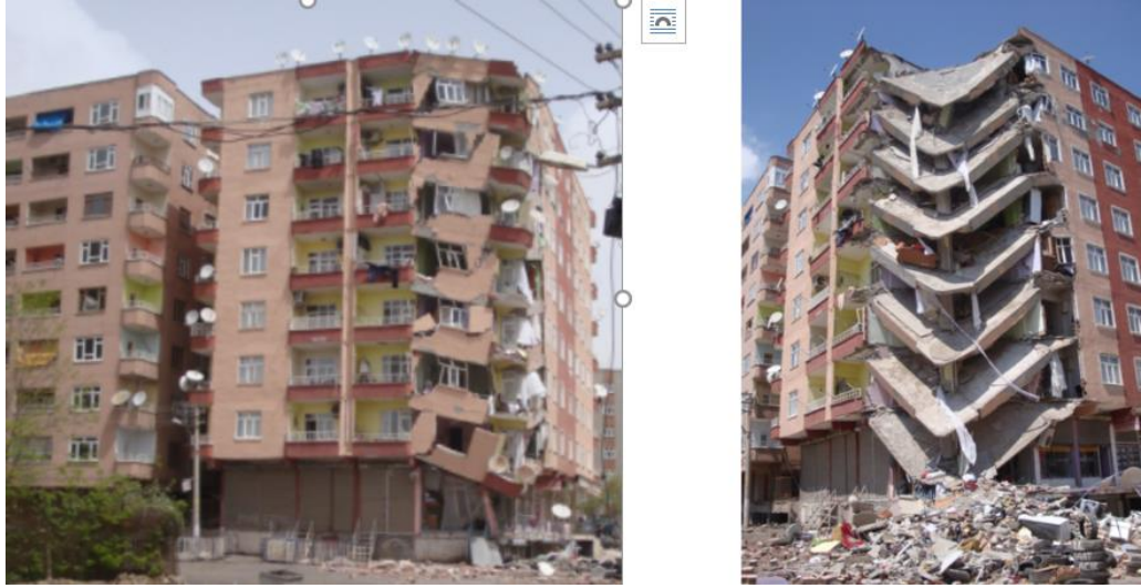
Figure1.2 The collapse of the building, which had damaged (Taken from the archive of Assoc. Prof. Dr. İdris Bedirhanoğlu, Bedirhanoglu 2011a)
