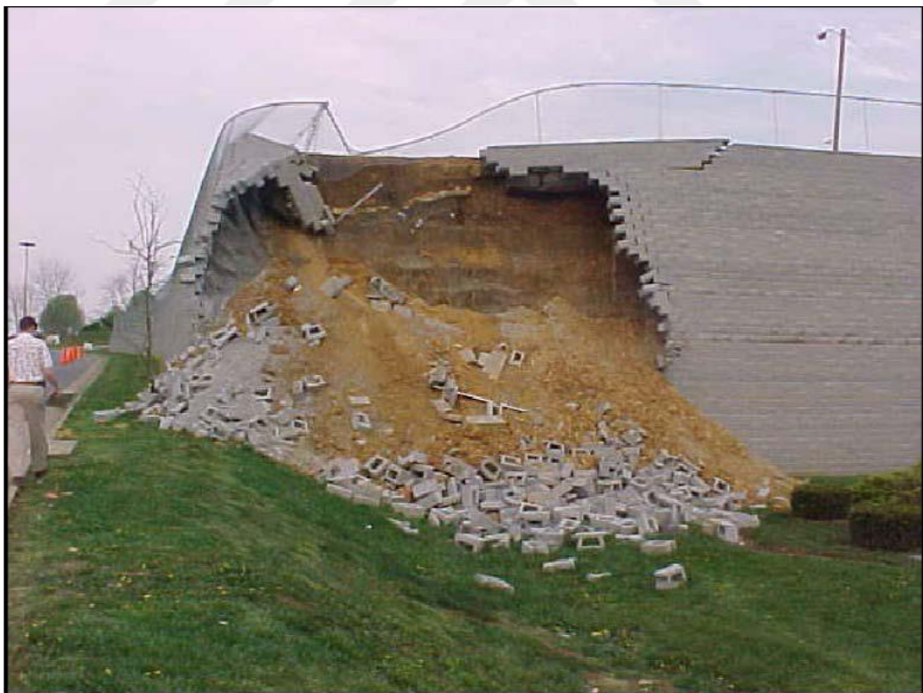
Figure 2.5. Failure of MSE wall due to lack of drainage and poor compaction of the reinforced fill soil [27].
