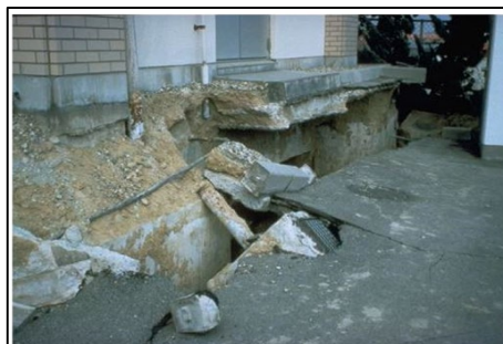
Figure 1.2: Soil Settling by Loma Prieta Earthquake San Francisco 1989.
