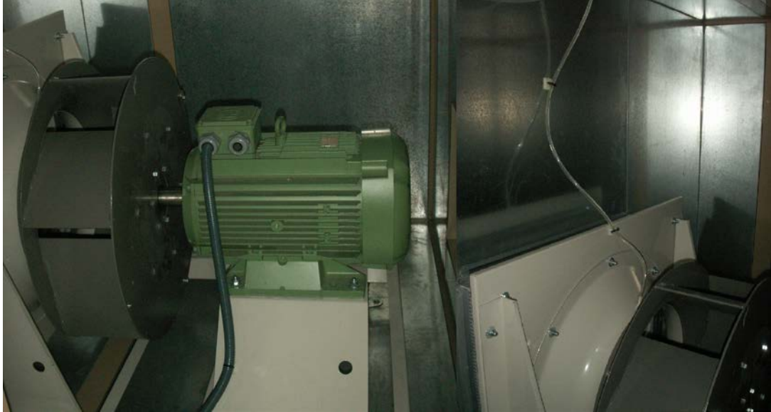
Figure 5.3 Plug fan speed control in cold air handling unit
