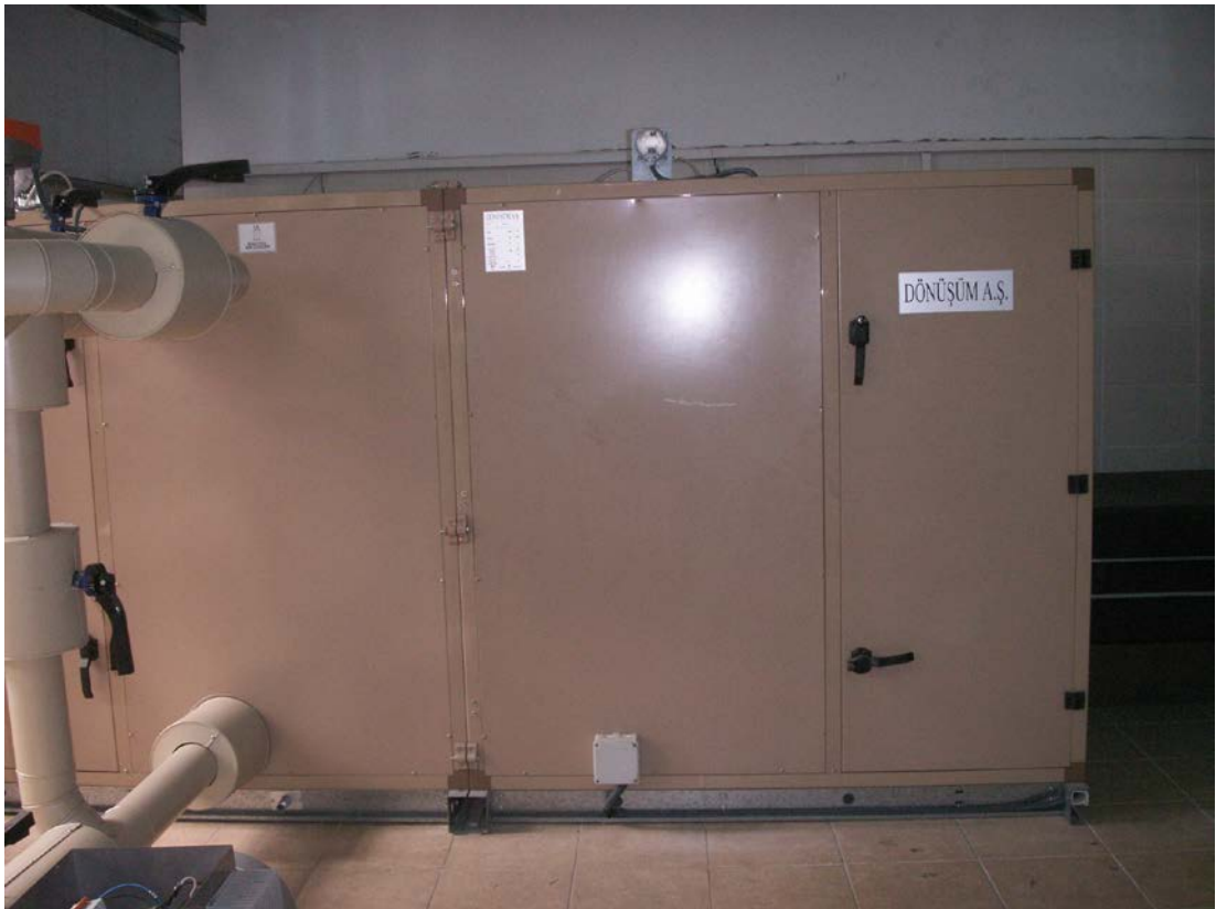
Figure 5.2 Cold air handling unit
