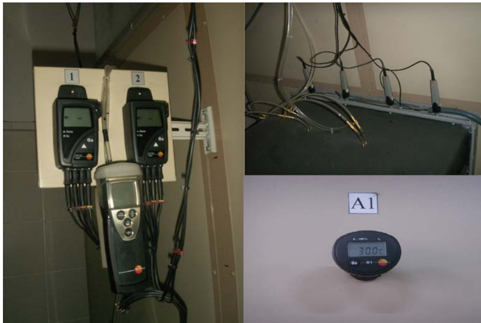
Figure 5.4 Manual temperature controls
