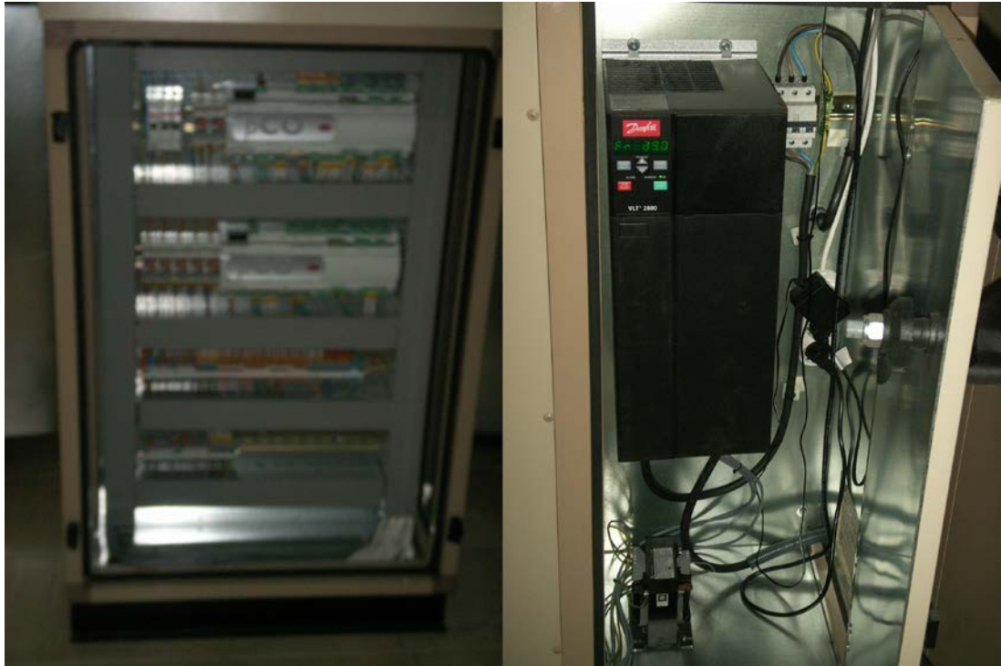
Figure 5.5 Microprocessor and air handling unit control panel
