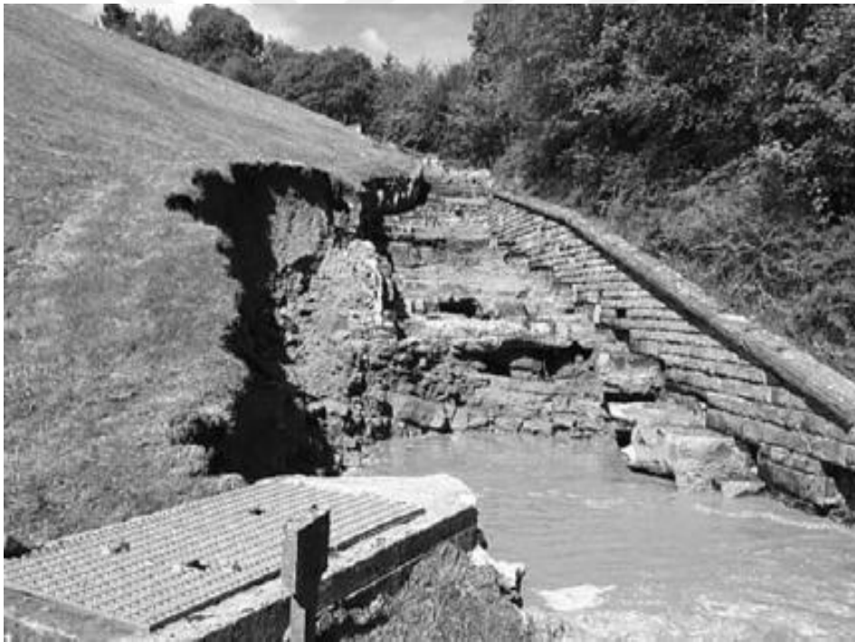
Figure 2.16. Flood event of June 2005 that resulted spillway damage at Boltby reservoir [4].
