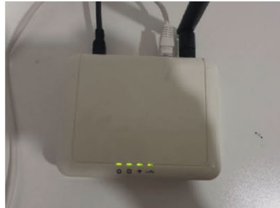
(b) Gateway of the indoor air quality sensors
