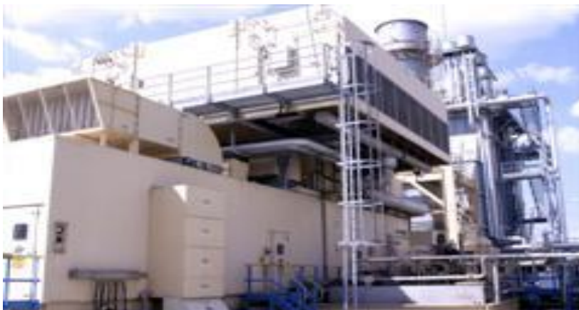
Figure 4.8 Ataer energy power plants in IAIP
