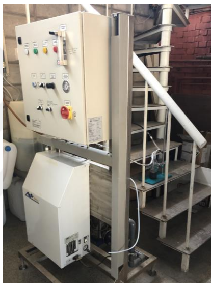
Figure 3.4. Ozone generator used in the study
