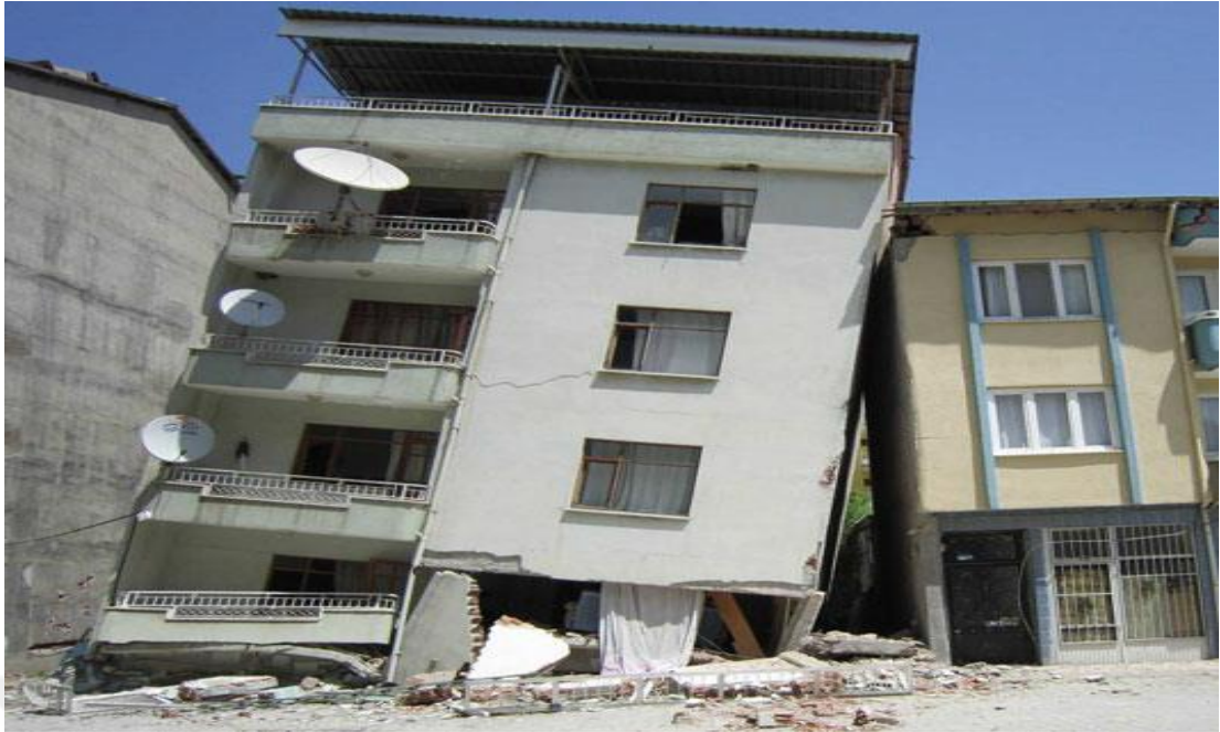
Figure 2.7 Totally collapsed building (Inel et al., 2013)
