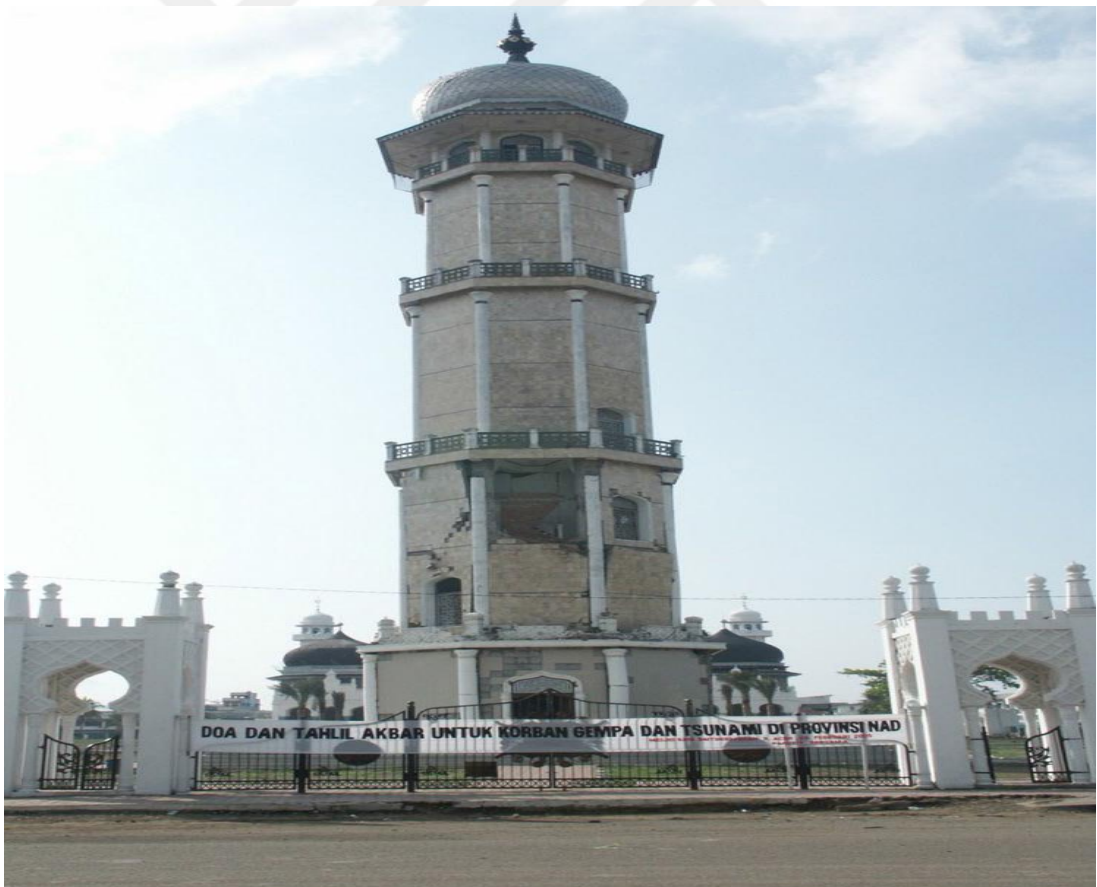
Figure 2.8 Earthquake damage to the minaret of the Grand Mosque in Banda Aceh (Ghobarah et al., 2006)
