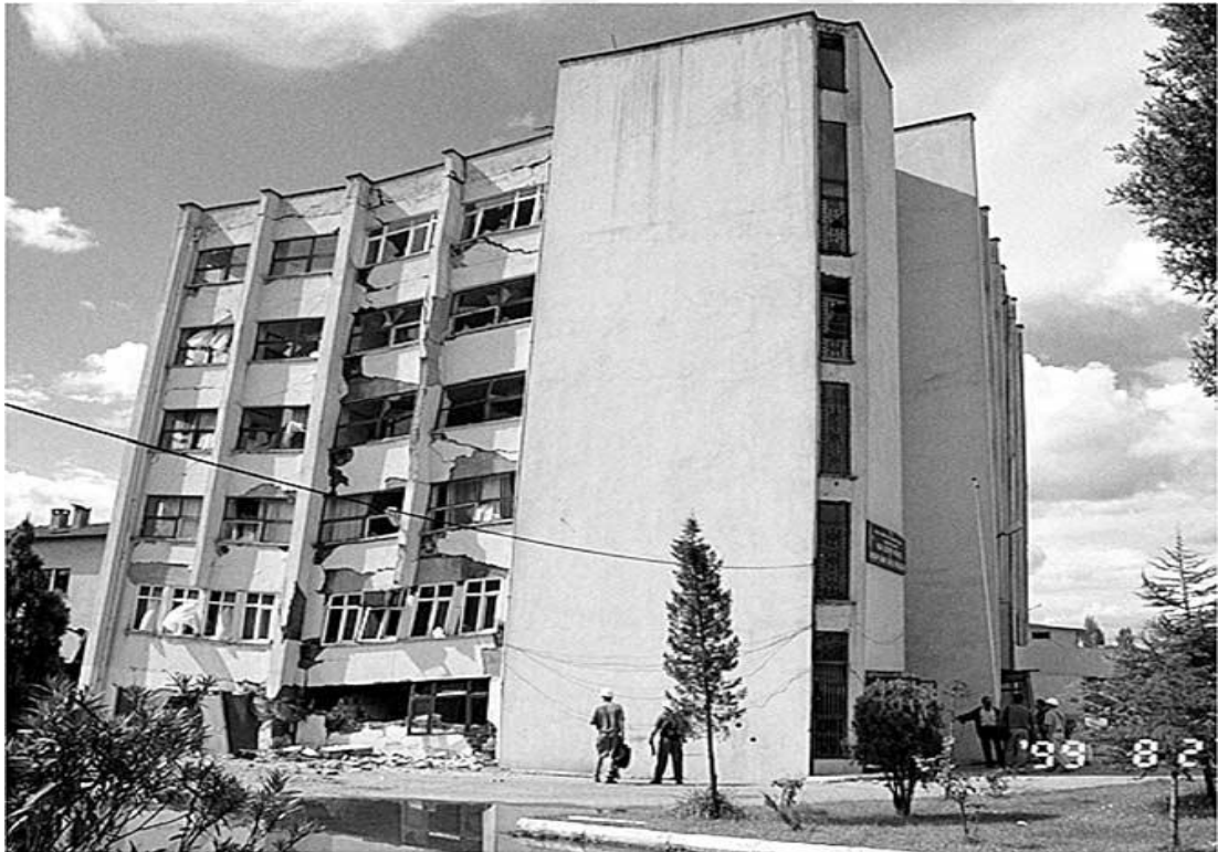
Figure 2.6 Damaged wall frame building due to ground failure and wall rotation (Sezen et al., 2003)
