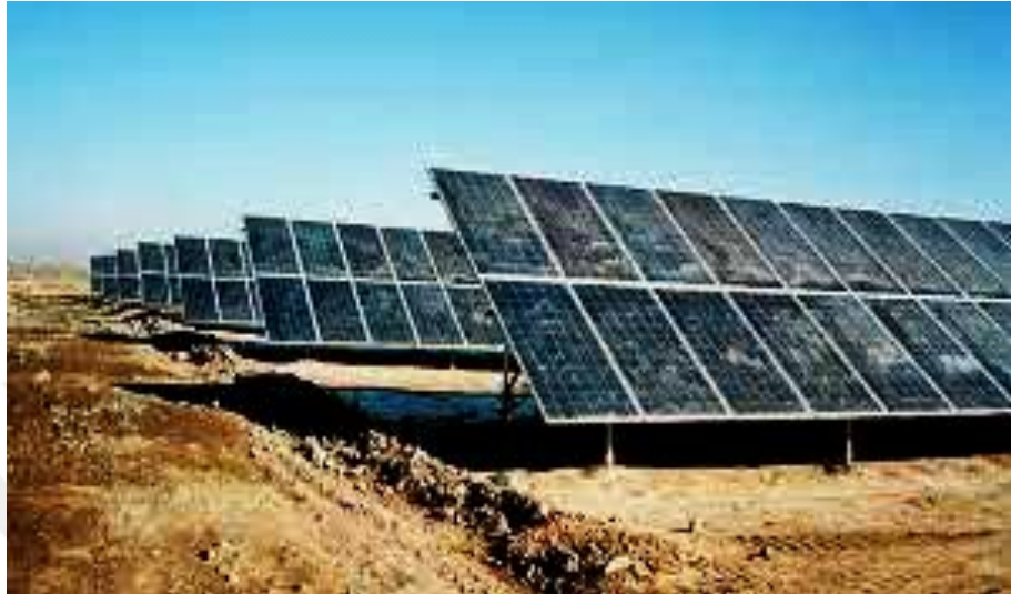
Figure 3.9 Amounts of dust that have accumulated on various PV modules that have been put in Iraq in an inclined arrangement.
