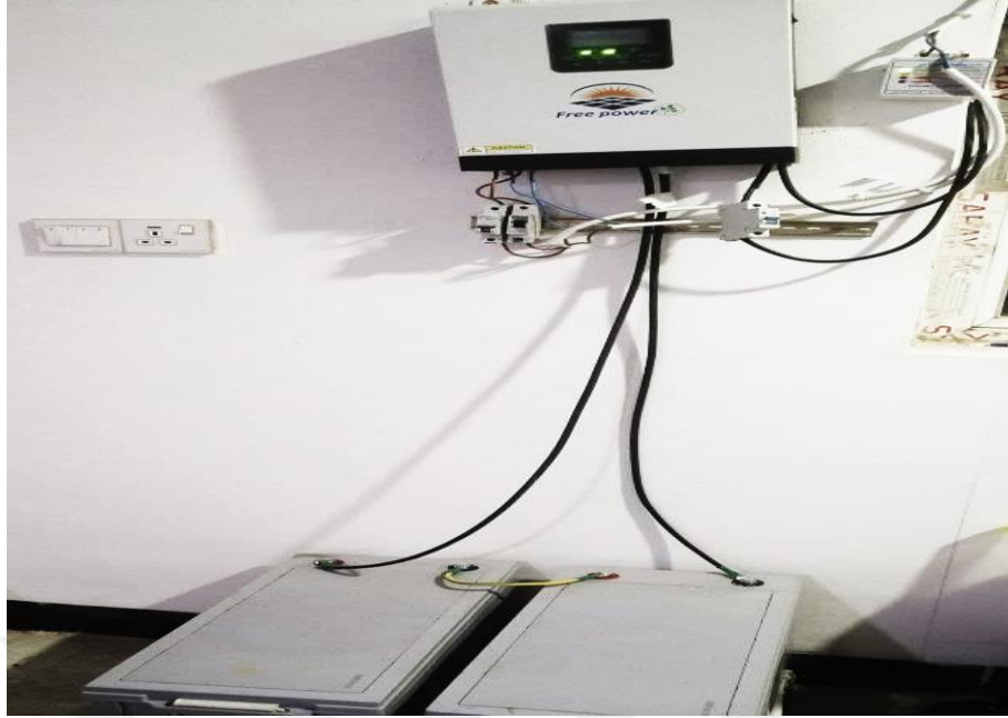
Figure 4.3 Full Solar system showing the invertor device and the batteries
