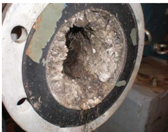
Figure 3.1 Scaling problems in pipes caused by struvite deposits (Bergmans, 2011)
