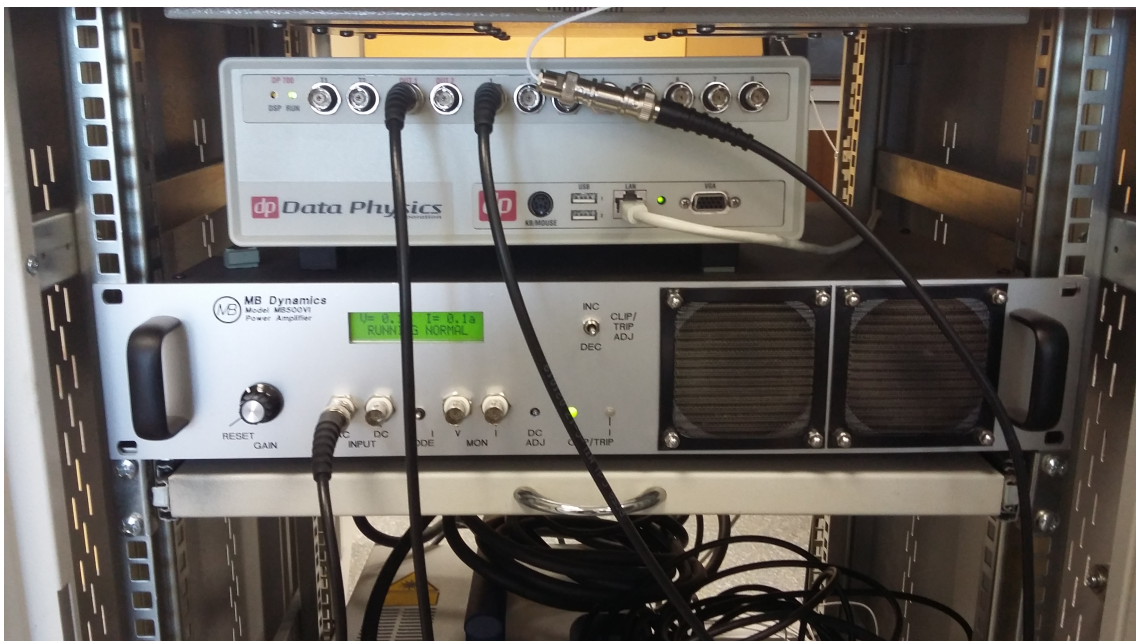
Figure 4.3: The controller and power amplifier
