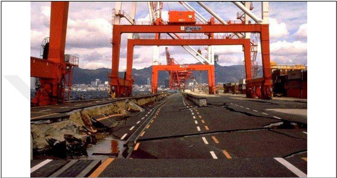
Figure 1.3. Kobe earthquake in Japan in 1995 [6]
