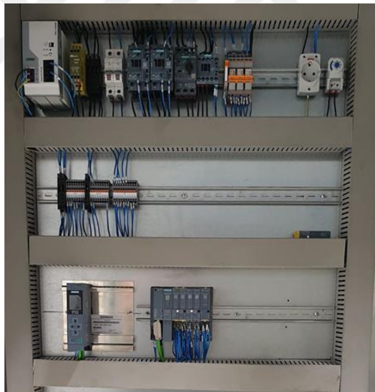
Figure 5.5 Electrical panel – control system (Personal archive, 2019)
