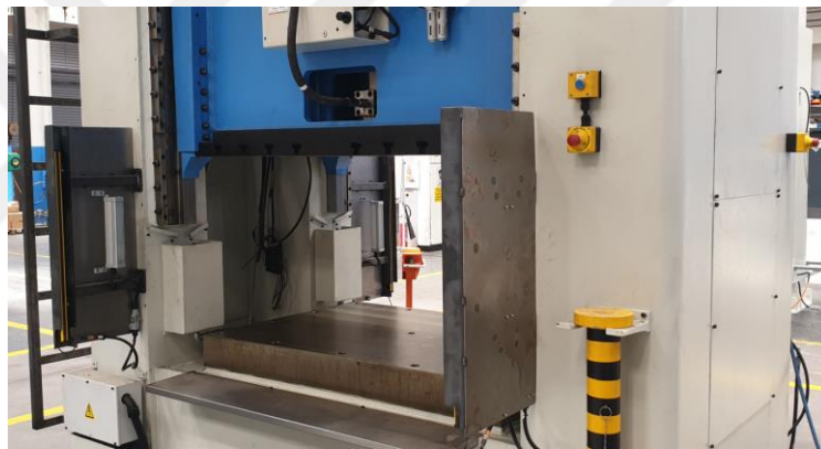
Figure 5.24 The emergency stop buttons that are placed at columns (Personal archive, 2019)
