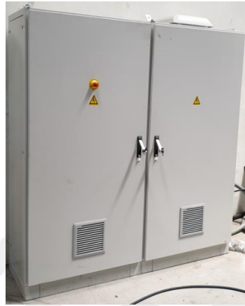
Figure 5.3 Electrical panel (Personal archive, 2019)
