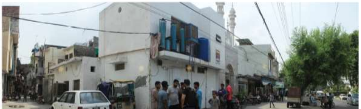
f. A collectively installed Water purification plant by the inhabitants of the Lal Quarter Settlement
