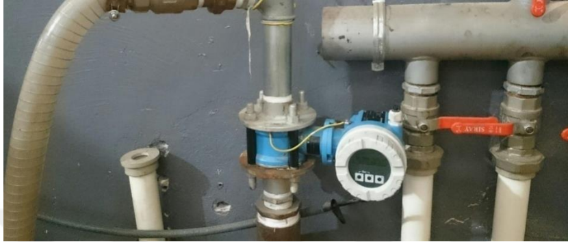
Figure 3.14: A photograph of the flowmeter.
