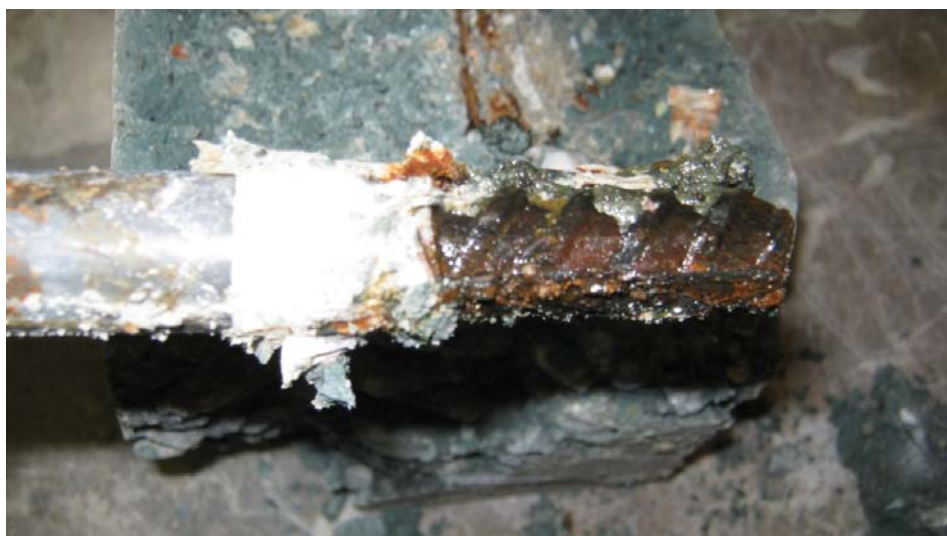
Figure 4.43: Obtained uniform corrosion along the length of a reinforcement bar.
