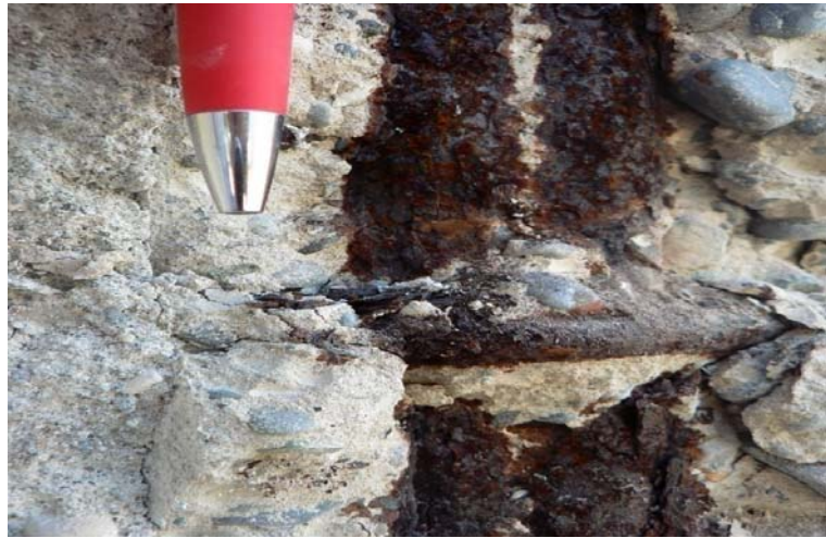
Figure 3.19: Outface of S 3 column.
