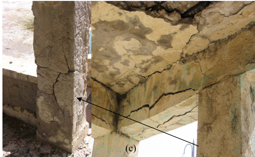
Figure 1. 2: Strength degradation due to corrosion: (a) Apostolo andreas monastery in Karpaz, 1985, (b) Corrosion rust in 35 years after construction, and (c) An old constructed RC building in Palmbeach.
