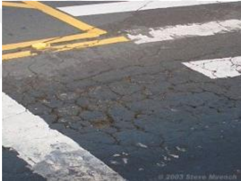
Figure 2.10 Severe alligator cracking near the stop line at an intersection (Hawai Asphalt, 2012)
