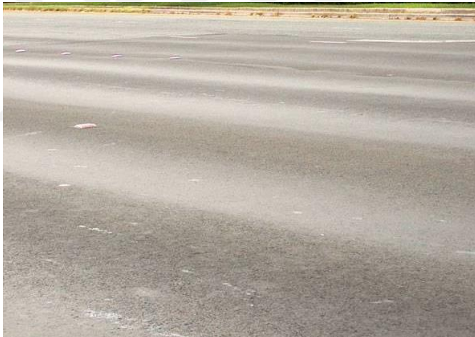
Figure 2.9 Shallow rutting (vertical indentation) is observable in this street (Pavement interactive, 2014)
