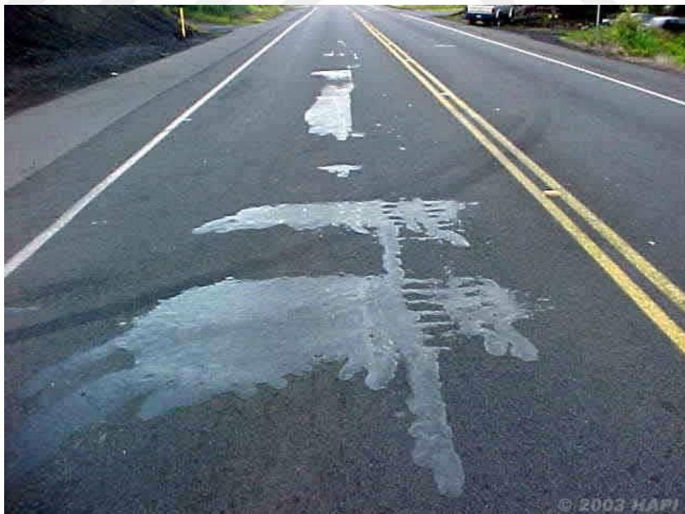
Figure 2.13 Severe bleeding (Pavement interactive, 2012b)
