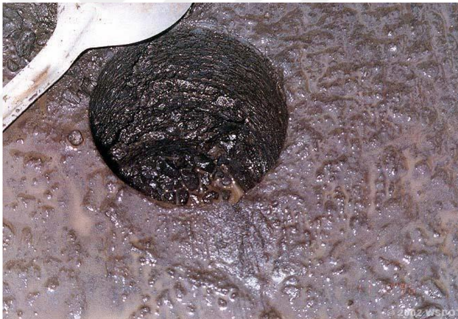
Figure 2.12 A small pavement core showing stripping at the bottom of the pavement section (Pavement interactive, 2012b)
