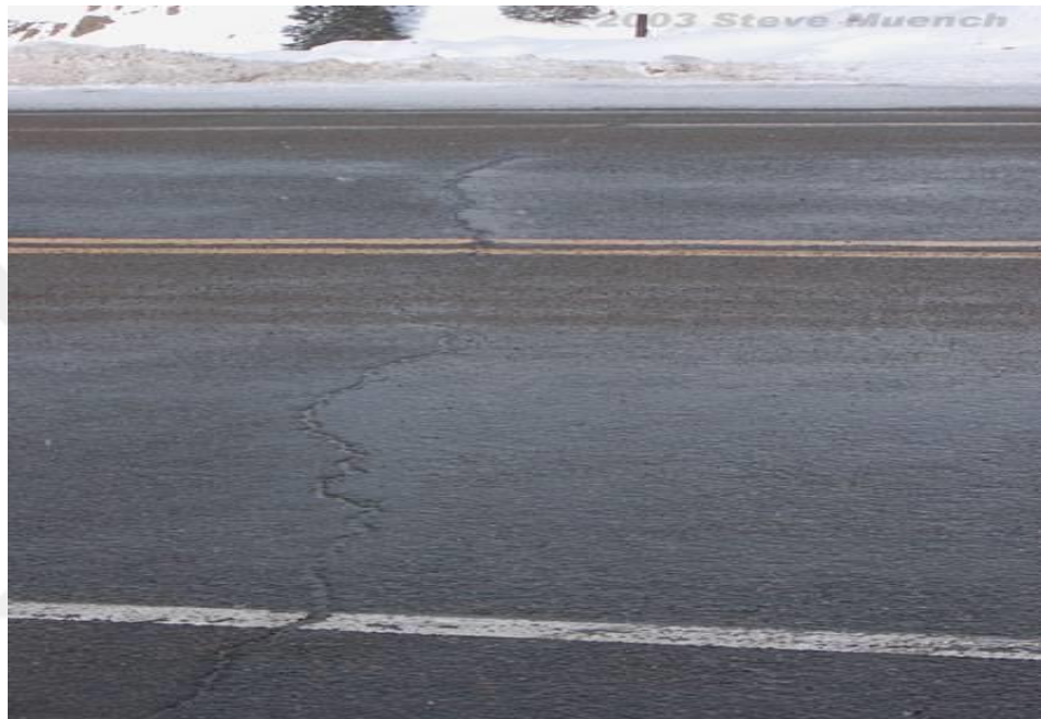
Figure 2.11 Transverse (thermal) cracking (Pavement interactive, 2012b)
