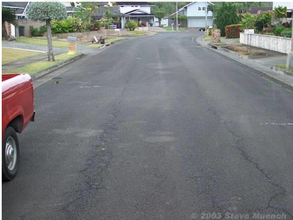
Figure 2.14 Longitudinal cracking (Pavement interactive, 2012b)
