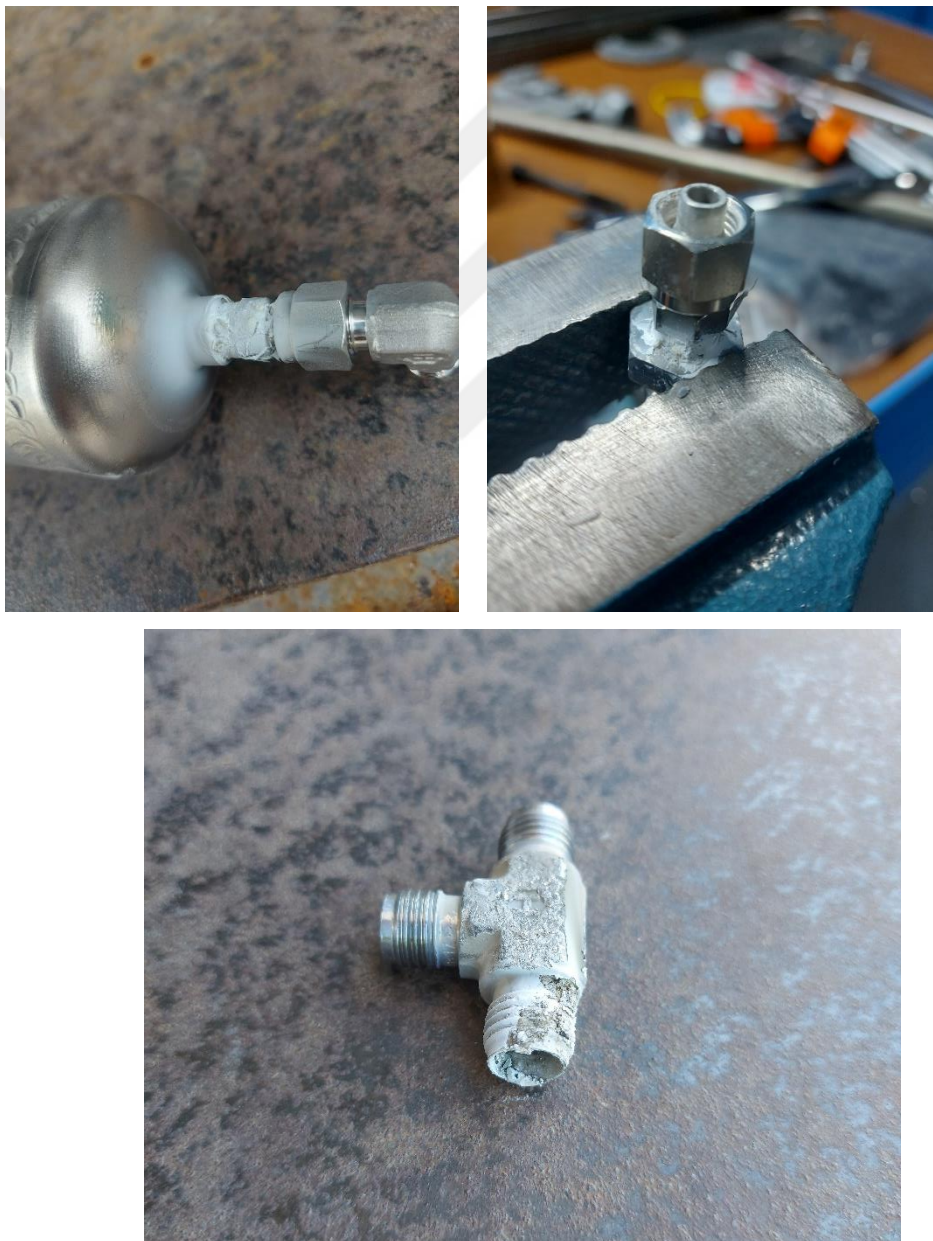
Figure 4.5: Fitting deformation due to leakage.
