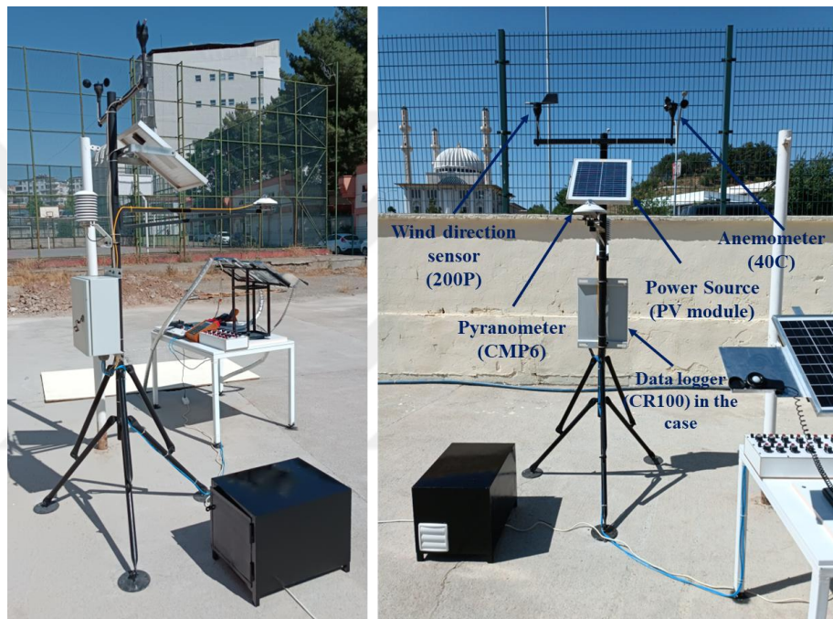
Figure 7.3. The meteorological station (back and front views)
