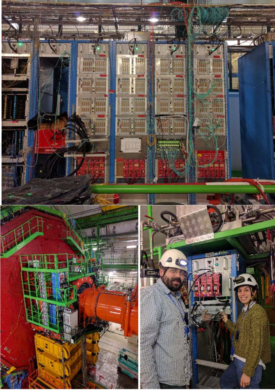
Figure 3.10. Photos from Phase-1 upgrades for the CMS HCAL. The HF burn-in test stand (top), including PMTs, FE and BE electronics. One of the HF cavern (bottom left). The bottom right photo from Installation and Commissioning of Front-End Electronics of the HF calorimeter
