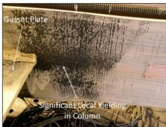
c) Local yielding in beam and column
