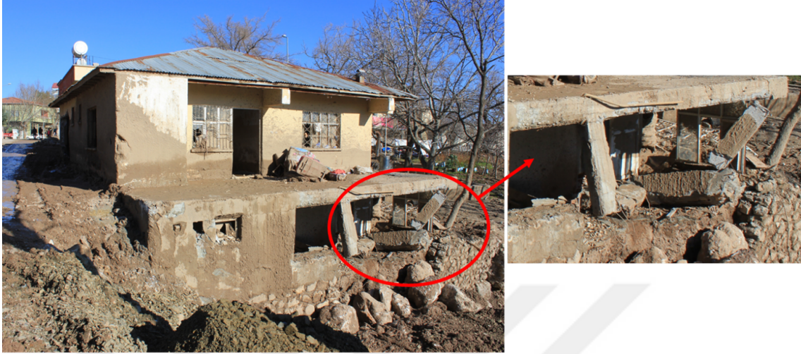
Figure 3.1: Damage to a reinforced concrete (RC) frame building due to flooding and flow-type landslide event in Adıyaman, Turkey (March 2023). The enlarged picture on the right highlights structural damage observed at the ground-floor columns[1].
