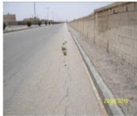
d) Yield crack
