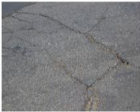
c) Block crack
