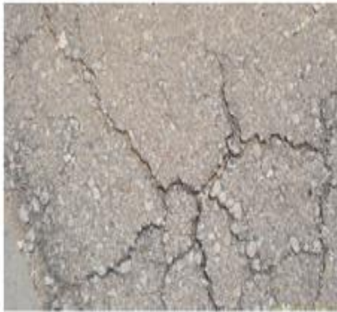
e) Spot ridge crack
