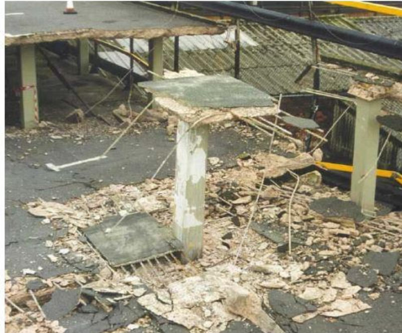
Figure 2.2 Punching shear failure in car park (Wood, 1997).
