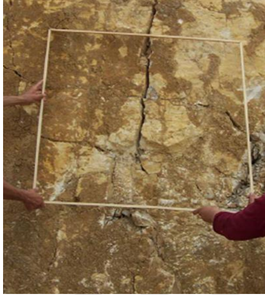
Figure 8.1 Photo showing the use of a square frame of 1 m of sides to measure the number of cracks on the benches (Personal archive, 2017)
