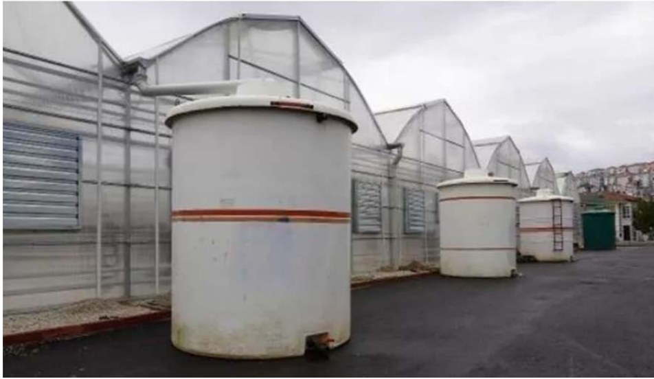
Figure 17. Steel water tanks
