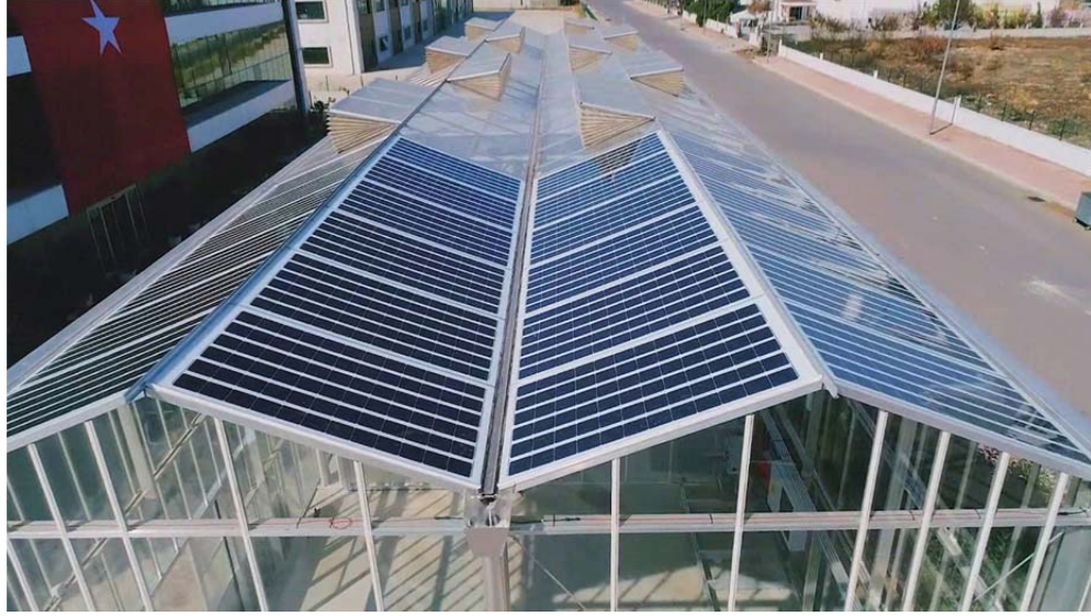
Figure 13. Solar Energy Panel
