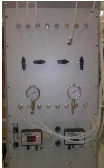
Figure 3.15: Cooling system rack panel.
