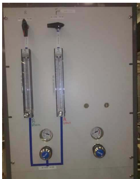
Figure 3.13: Active gas system rack panel.
