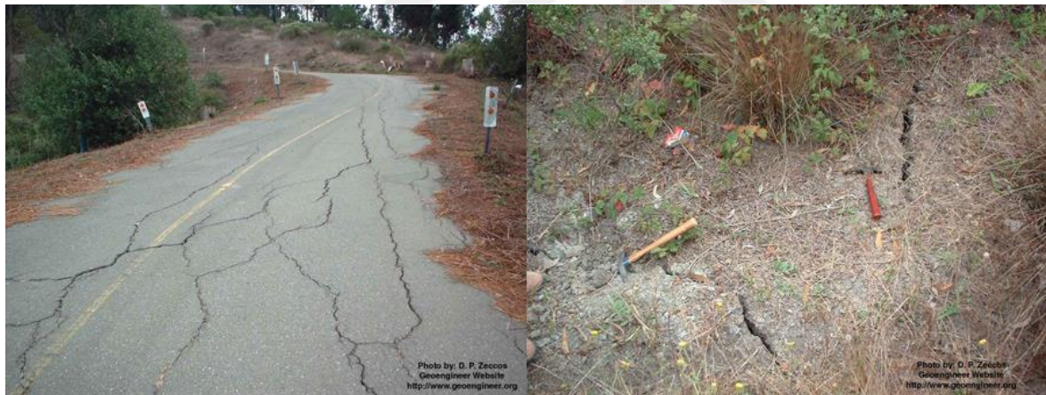
Figure 1.8. Cracks due to expansive soil (URL-1, 2021).
